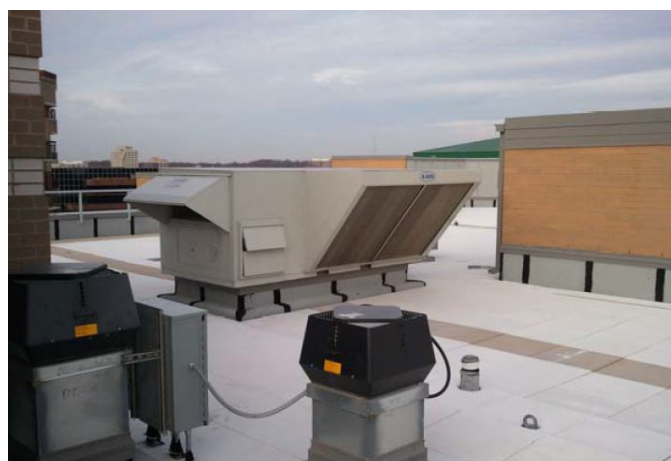
Dedicated outdoor air system
