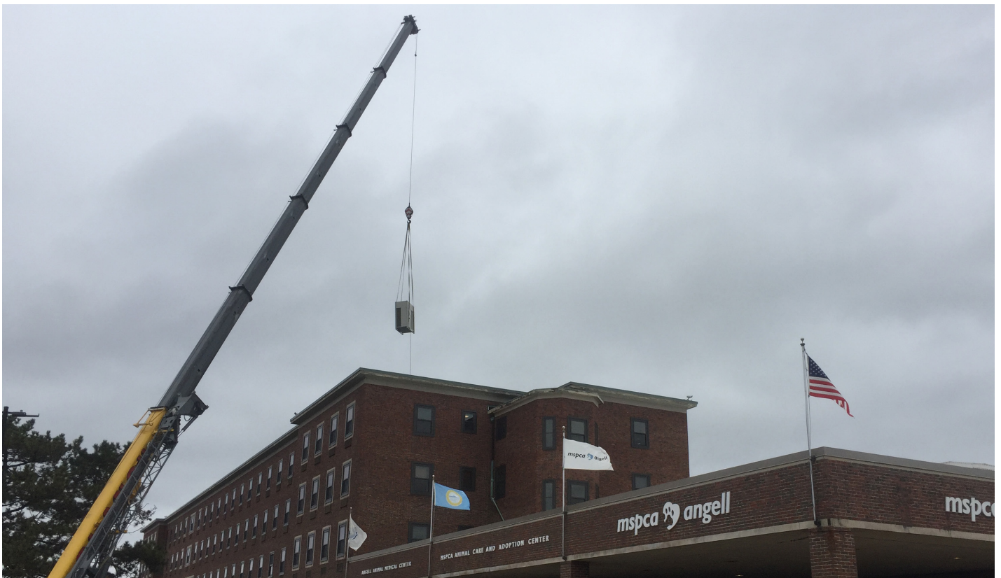
Air-source heat pumps are lifted onto the roof of the MSPCA-Angell Animal Medical Center in Jamaica Plain, Mass.
