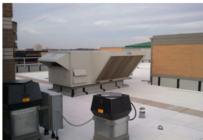
Dedicated outdoor air system
