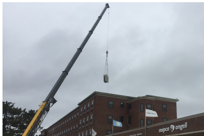
Air-source heat pumps are lifted onto the roof of the MSPCA-Angell Animal Medical Center in Jamaica Plain, Mass.
