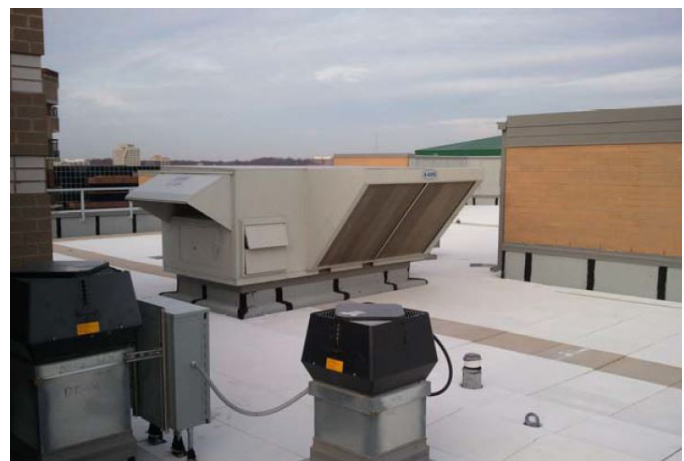
Dedicated outdoor air system
