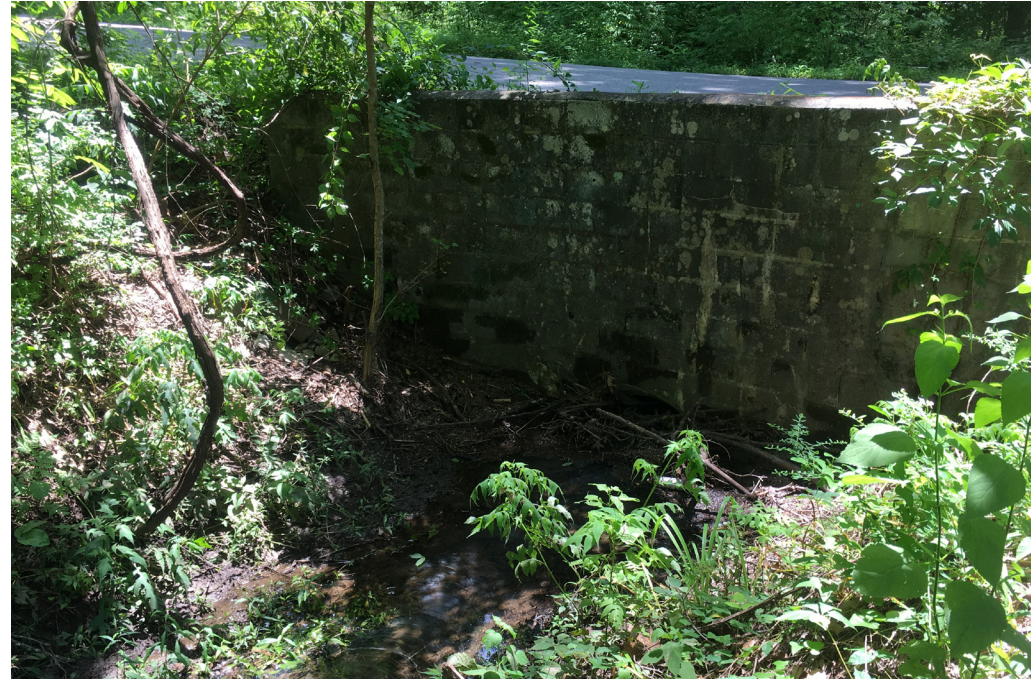
Figure 1-4: Partially Clogged Headwall South of Print Services Building.
