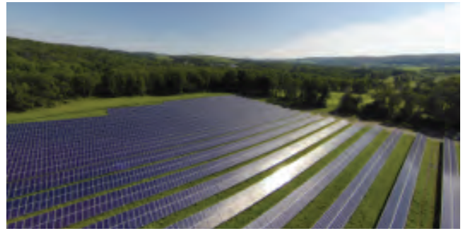
Millbrook School 1.7MW solar system located in Millbrook NY
