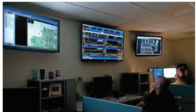
Real-time energy monitors at Princeton University
