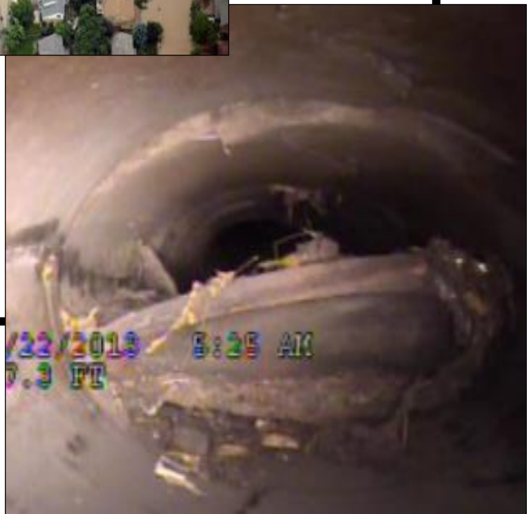
Image 1.0.2: Failed stormwater pipe
