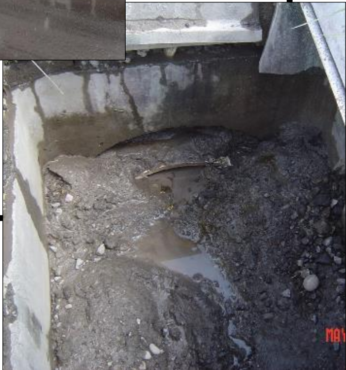
Image 5.0.2: Inlet sump clogged with construction debris
