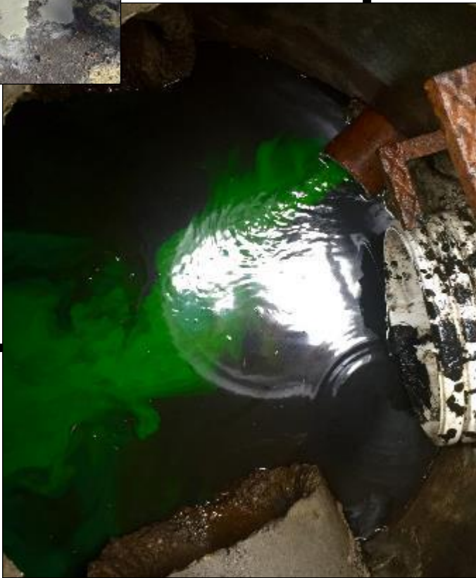
Image 4.0.2: Illicit connection confirmation through dye test
