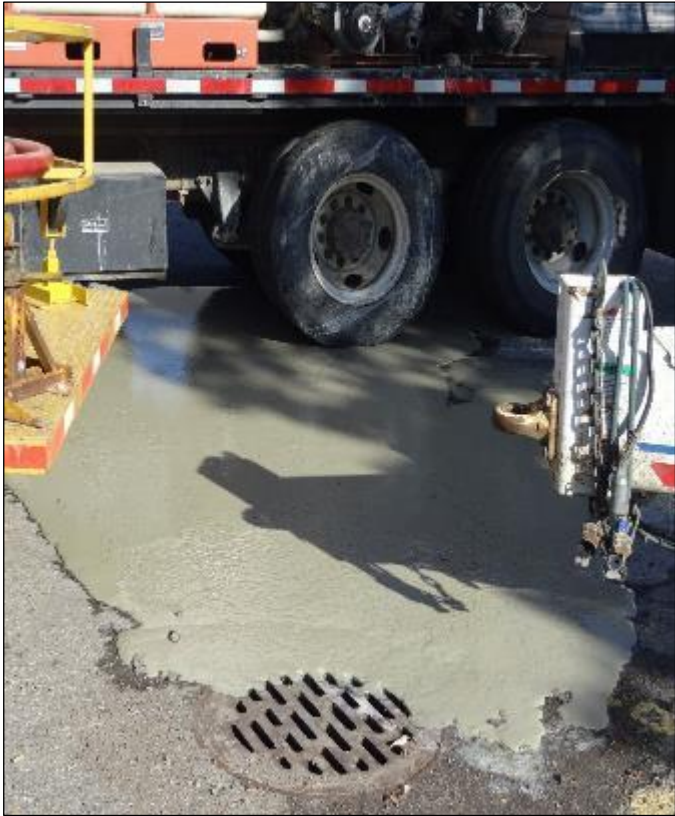
Image 4.0.1: Bentonite slurry spill
