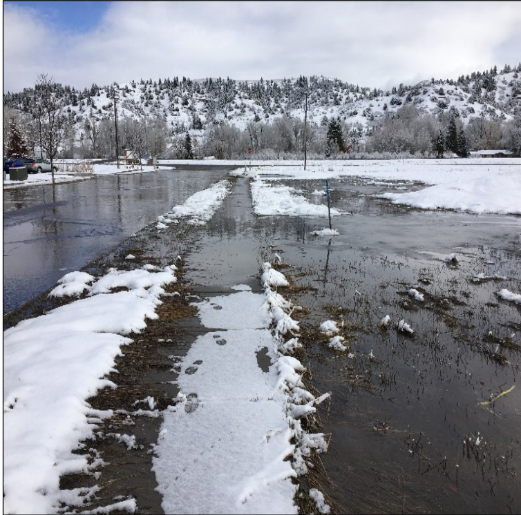
Graphic 1.0.1: Street-flooding resulting from clogged infrastructure
