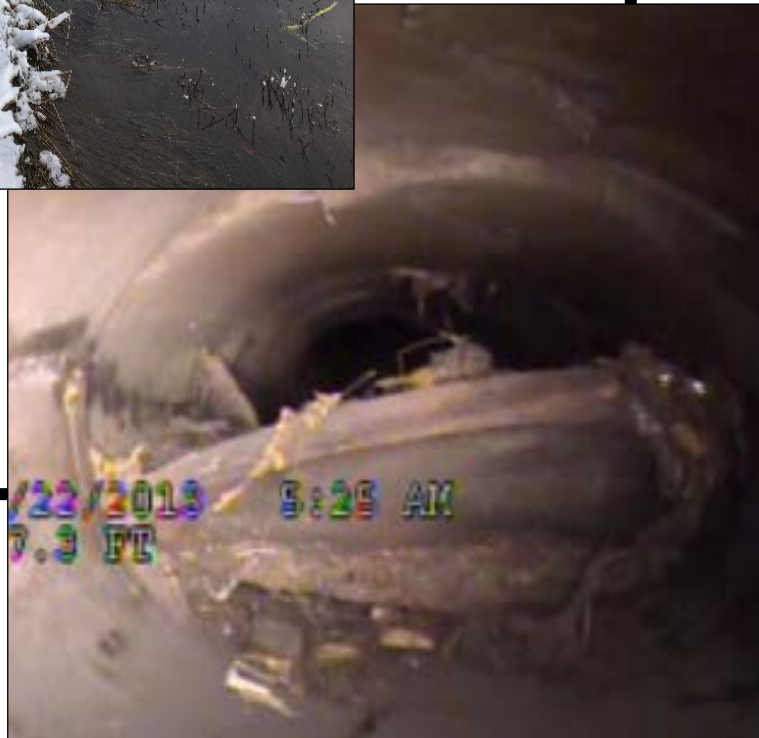
Graphic 1.0.2: Failed stormwater pipe
