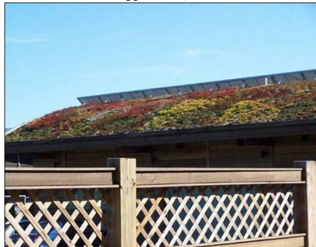
Figure 5.44 Green roof installed on a sloped roof, Tupper Lake, NY
