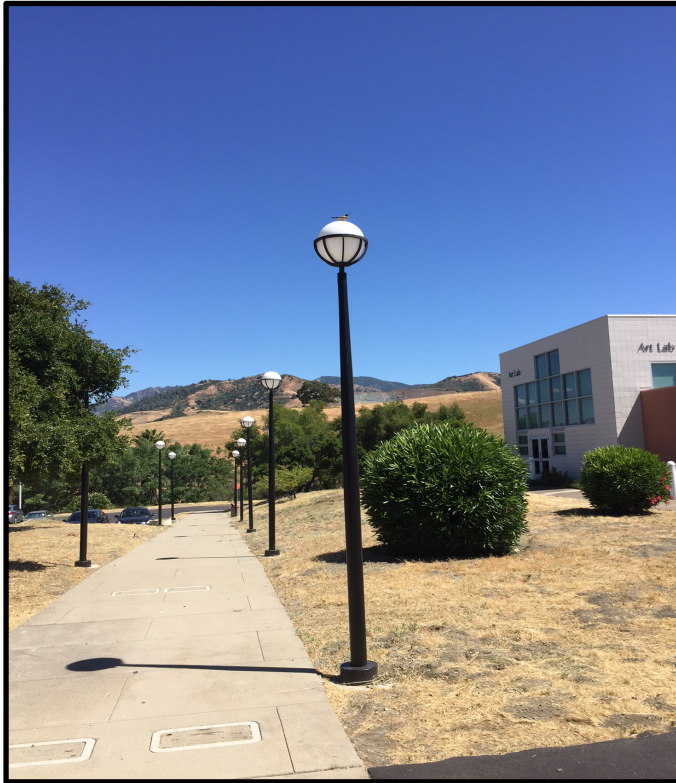
LED walkway lighting on the Concord Campus.
