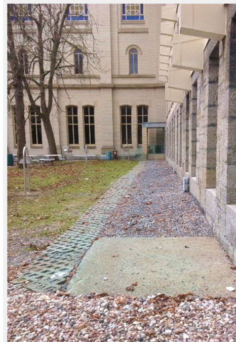
This photo illustrates green coloration caused by copper contamination from roof runoff.
