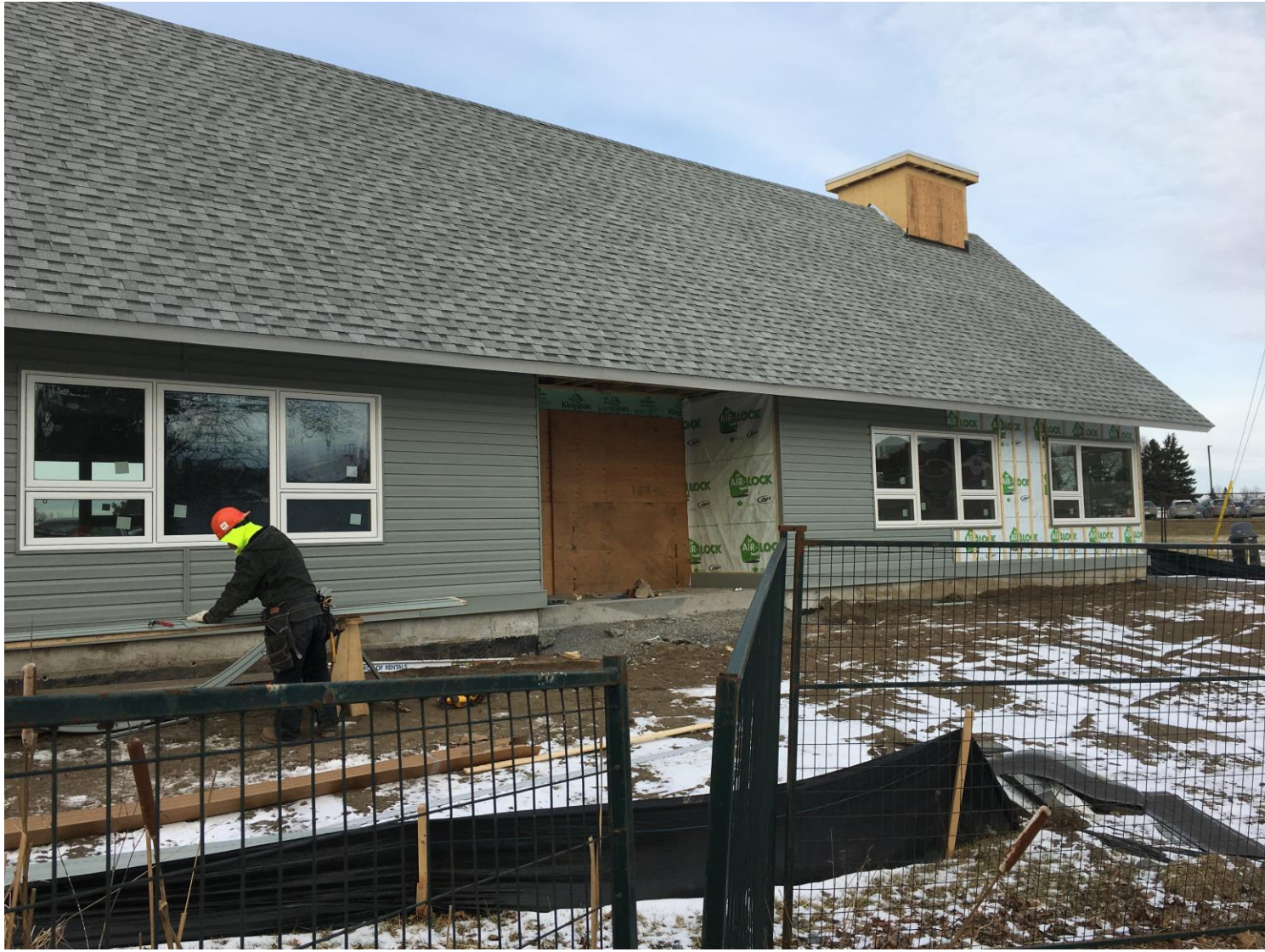
Figure 3. Photo of the south facing wall of the new Passive House project during its construction phase in mid January. (date of photo: January 17, 2019)
