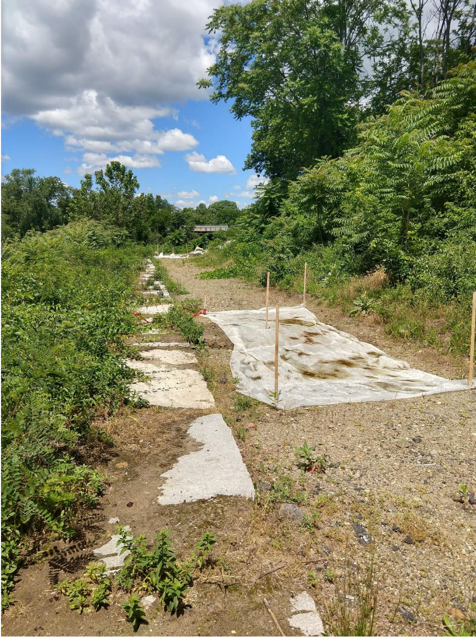
Figure 38: (North Campus Waypoint 11) Soil remediation project along the VFW highway and Merrimack River.
