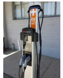
Electric Vehicle Charging Stations
