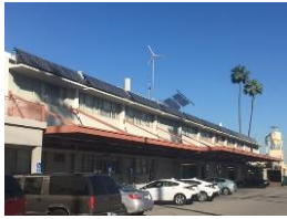
Solar PV System at E&T Building
