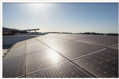
Some of CSUSM's buildings have solar panels installed on the roof, including the USU
