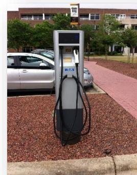
Plug-in electric vehicle charging station, Lot 17
