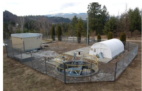
Figure 8. Effluent treatment centre, Castlegar campus
