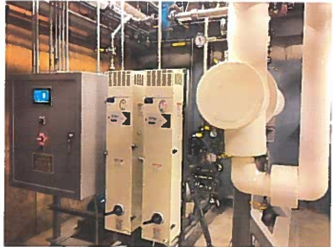
RFO Pump and Heating Skid
