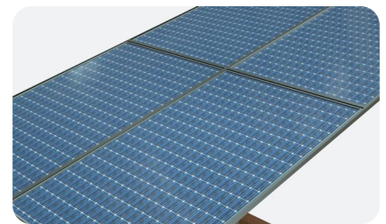
Powerful Solar Array
