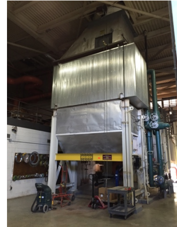
Inside CMU’s Power House
