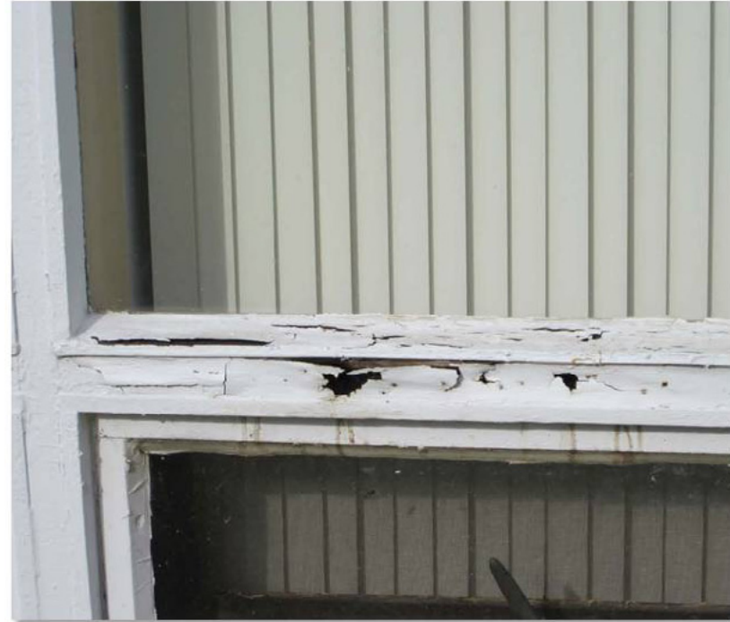
FAILING WOOD CURTAIN WALL, BARTLETT HALL
