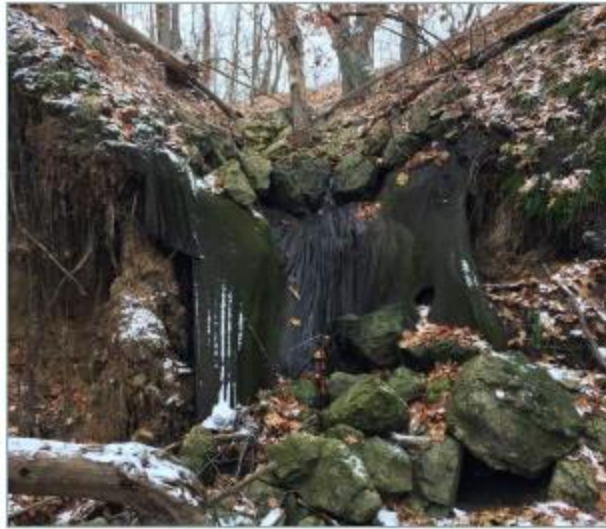
Failed stabilization measures in the Calder Ravine, Dec. 2021
