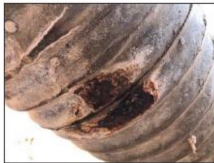
Deteriorating pipe – Au Sable
