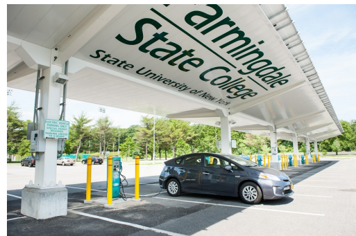
SUNY Farmingdale Solar Carport
