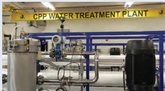
Cal Poly Pomona water treatment plant
