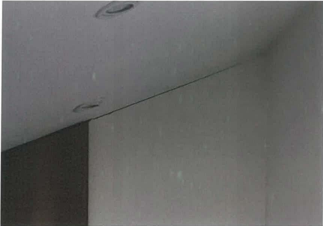
Foto 5 – Fisura identificata in perete – dormitor mansarda (07.01.2021)
