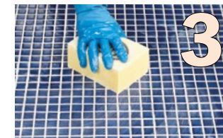
Wash any residue off the face of the tiles when slightly hardened in the joints, and up to 60 minutes after application
