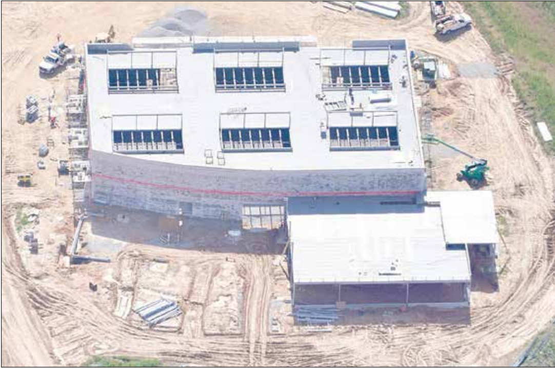
Commonwealth Crossing Business Center takes shape with construction of the Commonwealth Centre for Advanced Training (CCAT) building.
