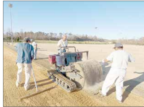
A crew worked on the SRSC fields before the sports complex's 2009 opening. Now, after 10 years of use, the turf on some fields will be replaced.
