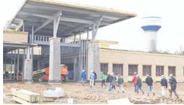
Tour participants enter the Commonwealth Centre for Advanced Training (CCAT) building. Construction of the facility is expected to be completed by early summer.
