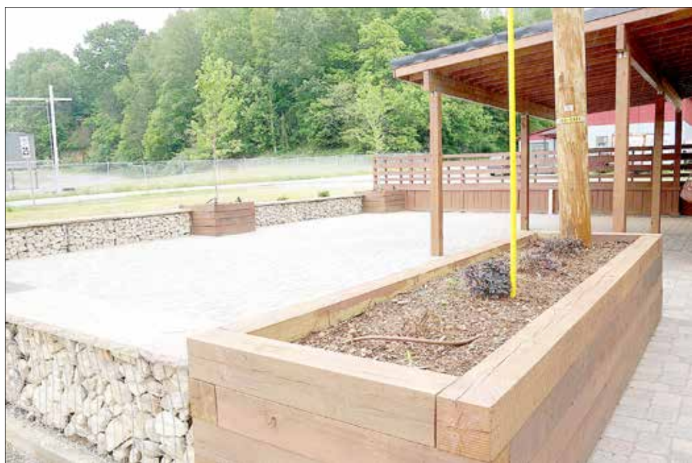
A patio area on one end of the Reed Stone Block has been created with a paver foundation, gabion seating walls, planters and partial roof. Inside, there are provisions for a kitchen, heating and air conditioning and other features.
