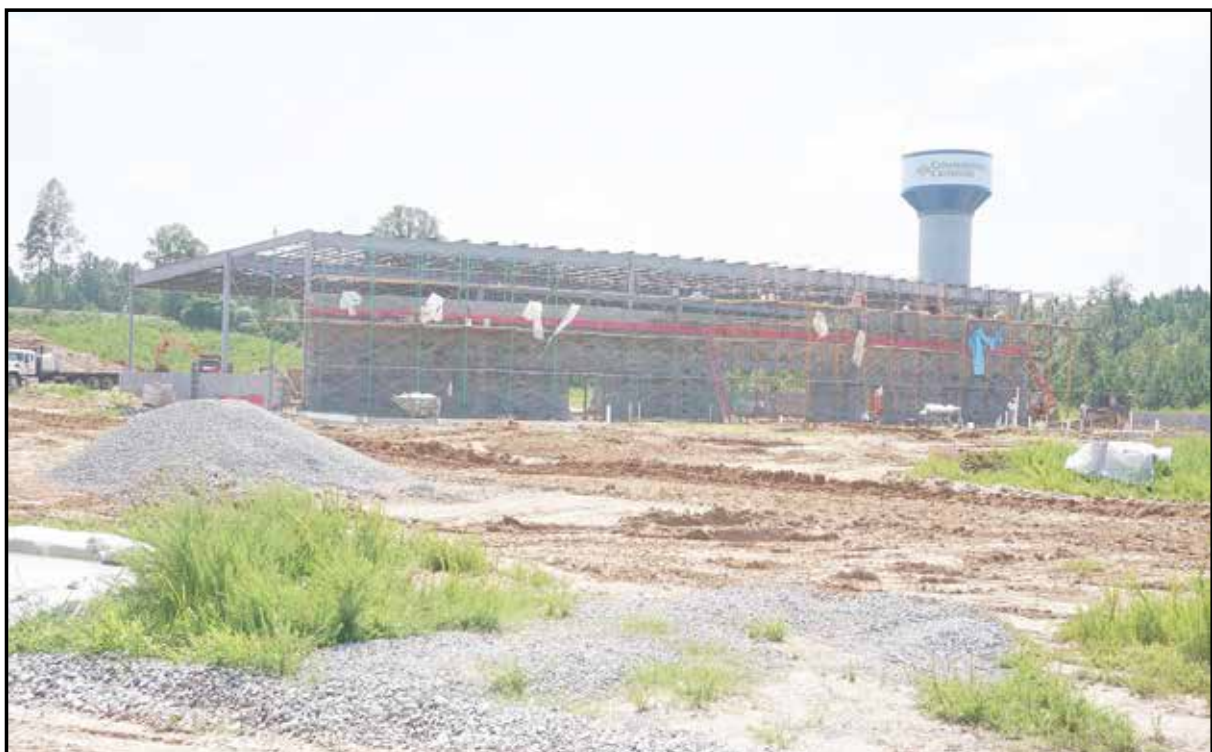
The CCAT training center takes shape at CCBC. The 25,500-square-foot building is expected to be open by next June. It will feature advanced manufacturing training facilities. (Contributed photo)
