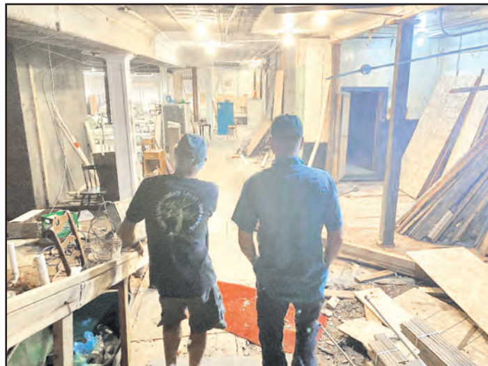
Herb Atwell (left) showcases the basement of the former Daystar building on Franklin Street in Martinsville. He and his wife, Peggy Donovan, who currently own Mountain Valley Brewing in Axton, plan to open up a new brewpub in the building in 2023 after extensive renovations are completed.
