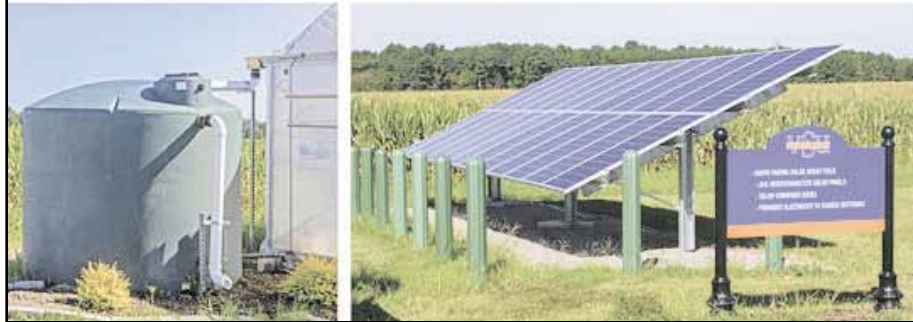
Clockwise from top left: Grace Summers leads a tunnel tour; VSU's Bill Crutchfield goes over the tunnel control panel; A 24-panel solar array helps power all tunnel functions; Cisterns conserve rainwater running off the tunnel roof.
