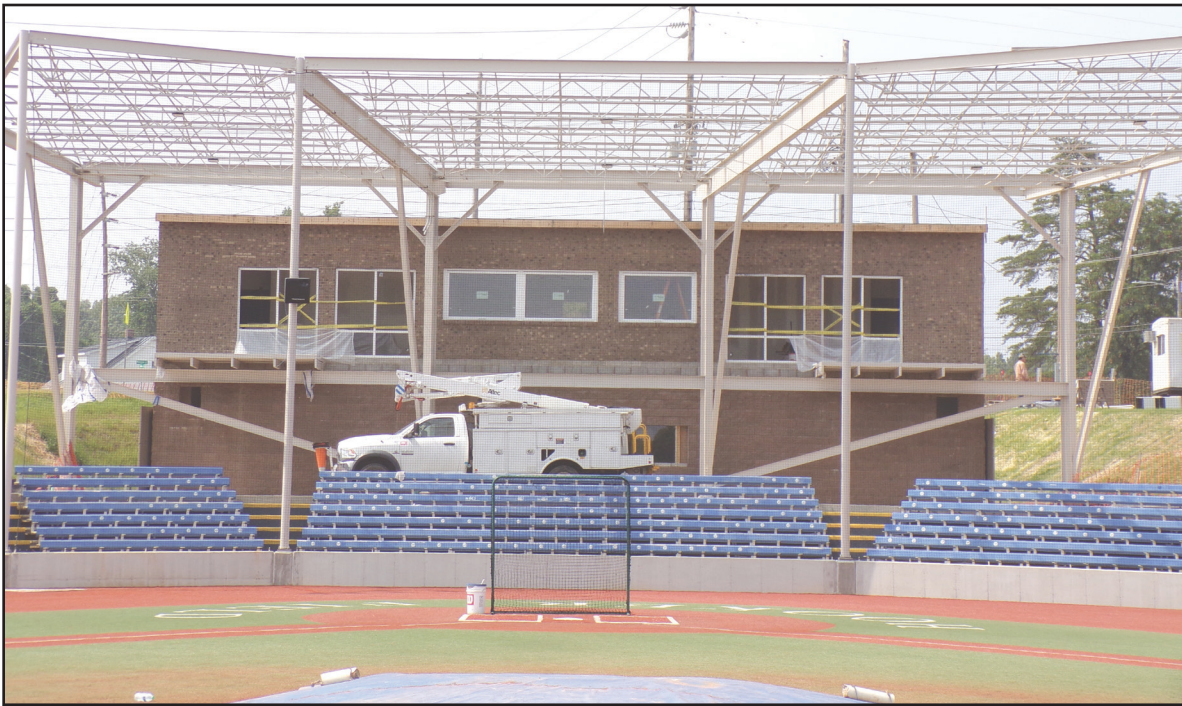
A view of the renovations to Hooker Field. Pictured is the area behind home plate, including the larger press box, concessions, new restrooms, and covered seating.
