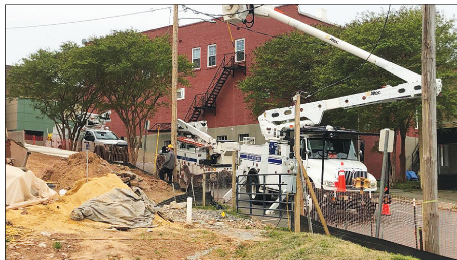
Electric lines were being installed Wednesday at the annex. Construction should be completed in May, and then it will take several months to get the displays established, under the direction of experts from the Virginia Museum of Natural History.
