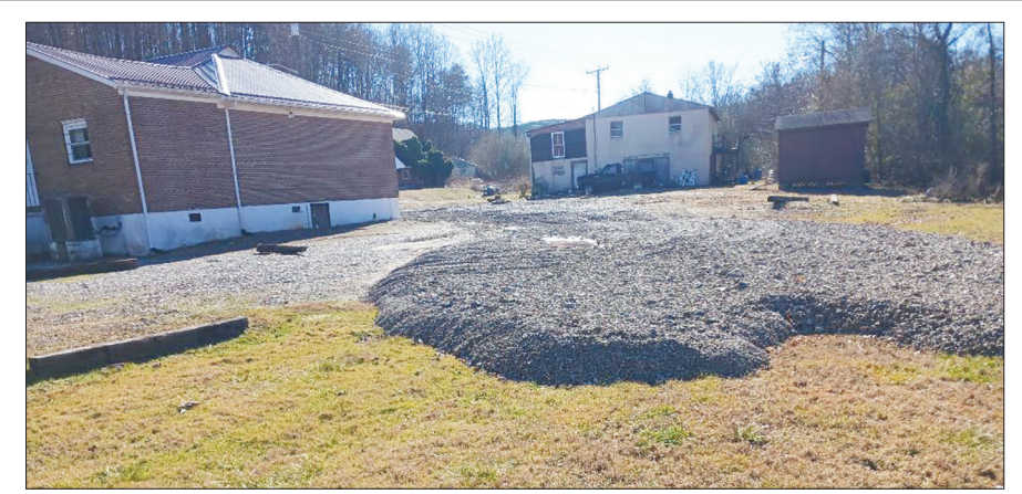
American Legion Homer Dillard Post #78 is seeking donations to repair flood damaged areas to its building. (Contributed) A video also is posted online at www.henrycountyenterprise.com.
