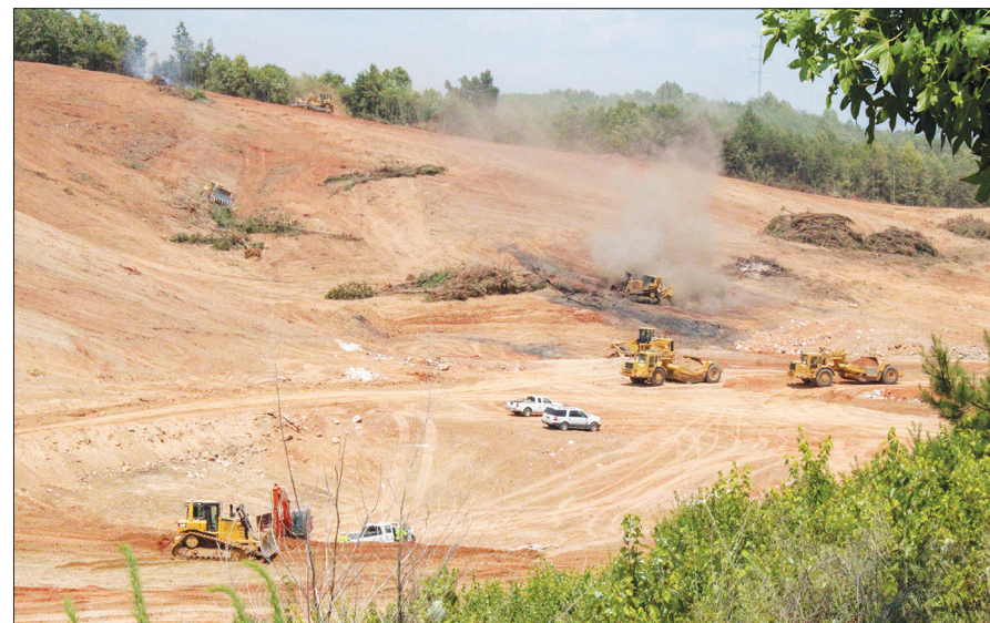
Grading work is underway on Tract 2 of the CCBC. As of Tuesday, about 57 of 150-acre pad have been graded.
