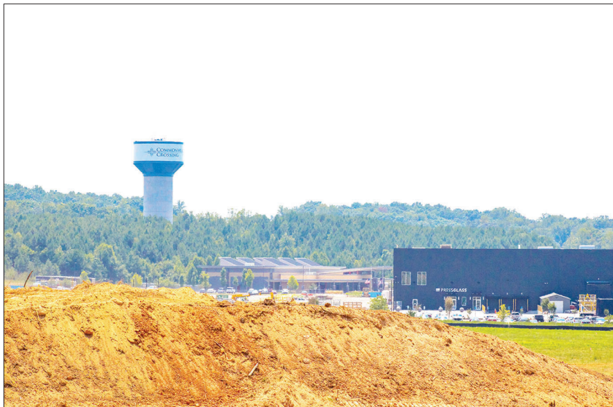
Tract 2 is situated near the operations of Crown Holdings, Inc. and Press Glass, Inc.
