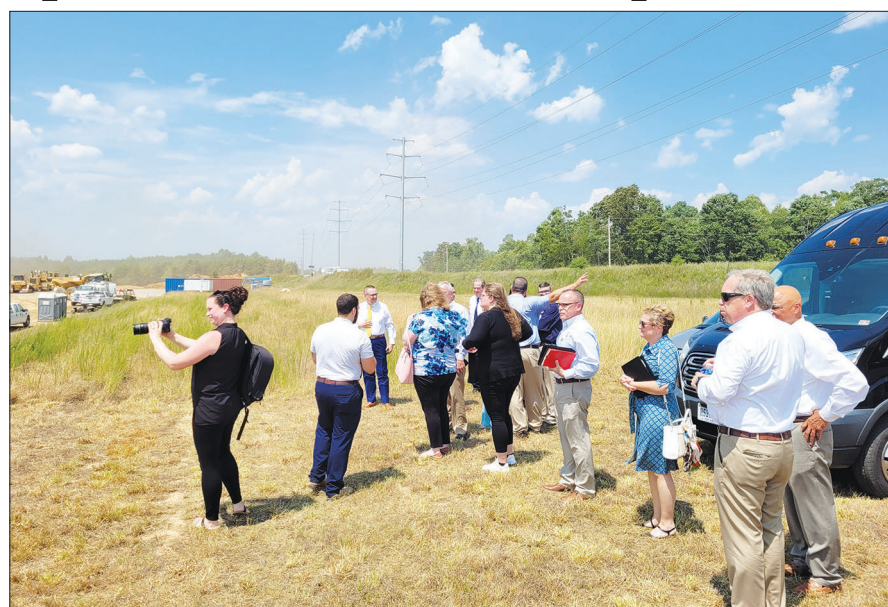
Local and other officials watch from the back side of Tract 2 as grading work continues.
