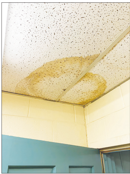
Ceilings on the first floor of Martinsville's Municipal Building sustained damage due to an HVAC leak, prompting the temporary relocation of the General District Court judge and clerk's offices.
