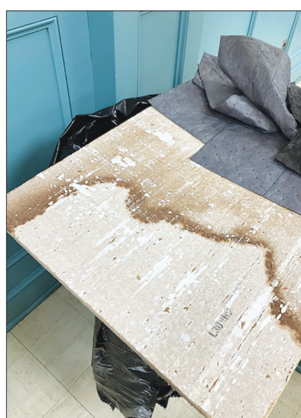
A water leak from condensation on HVAC pipes damaged ceiling tiles, causing some to fall. The tiles will be removed as the city works to address the issue.
