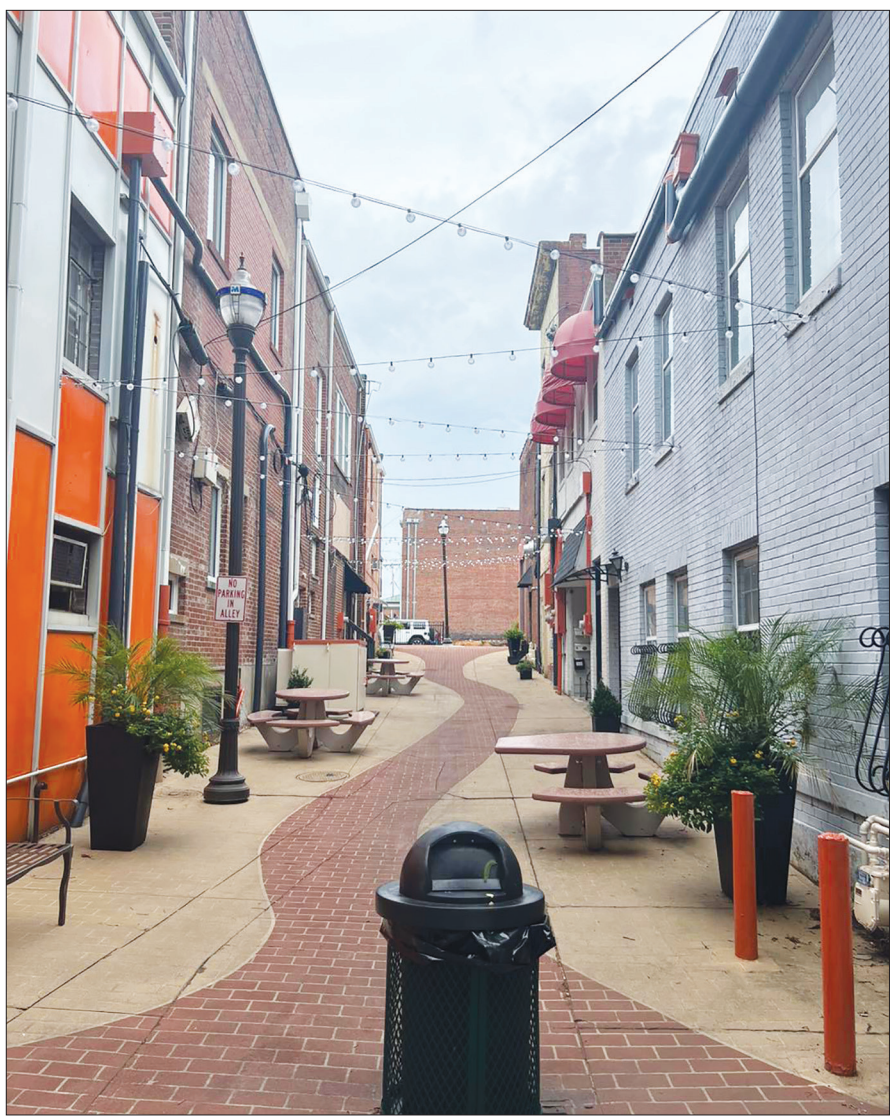
The Uptown Partnership announced that the Wall Street Alleyway now has lights. Reed Electrical Solutions helped with the installation.
