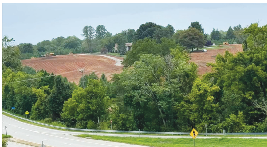
A solar facility is being built on the former Bassett Country Club property. (By Ray Reynolds)
