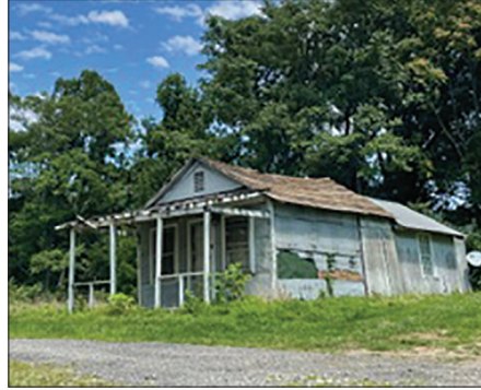
The humble abode known to many local residents as Blind Man Martin's house is pictured before it was demolished to the last splinter as work on the U.S. 58 project continued its march.
