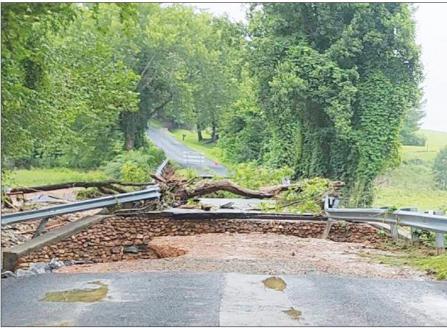
Floodwaters damaged the Rabbit Ridge Road bridge over the Ararat River. This photo was taken from the North Carolina side following flooding that began Aug. 1 and continued into Aug. 2. (Contributed by Mary Dellenback Hill)
