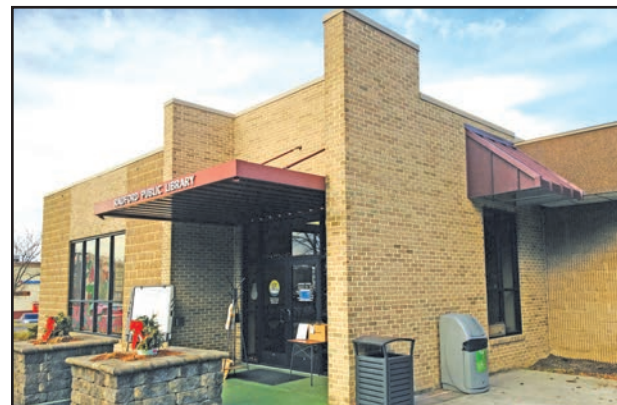
Walk-up window modifications are in progress at the Radford Public Library. The plan is to offer a walk-up service to accomplish things like faxing, copying, scanning and more. The overhang has been mounted and progress has been made, but it is not quite finished. Patrons can continue to call to make an appointment when services are needed.
