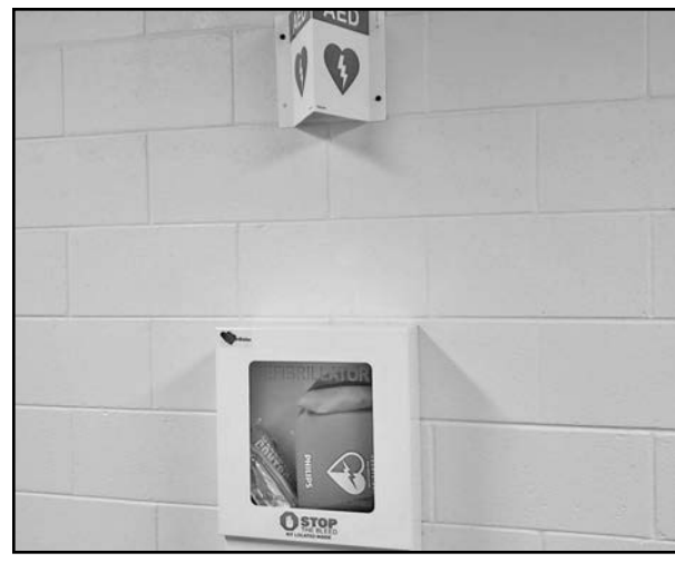
AED station located on the first floor of the Public Safety Building.
