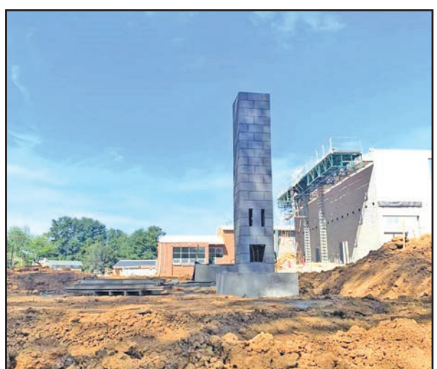
The Chimney Swift tower is now under construction on the grounds of McHarg Elementary School.
