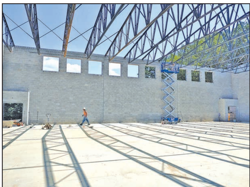
The large floor plan of the new gymnasium can be seen against the backdrop of the worker walking along the far wall of the structure.
