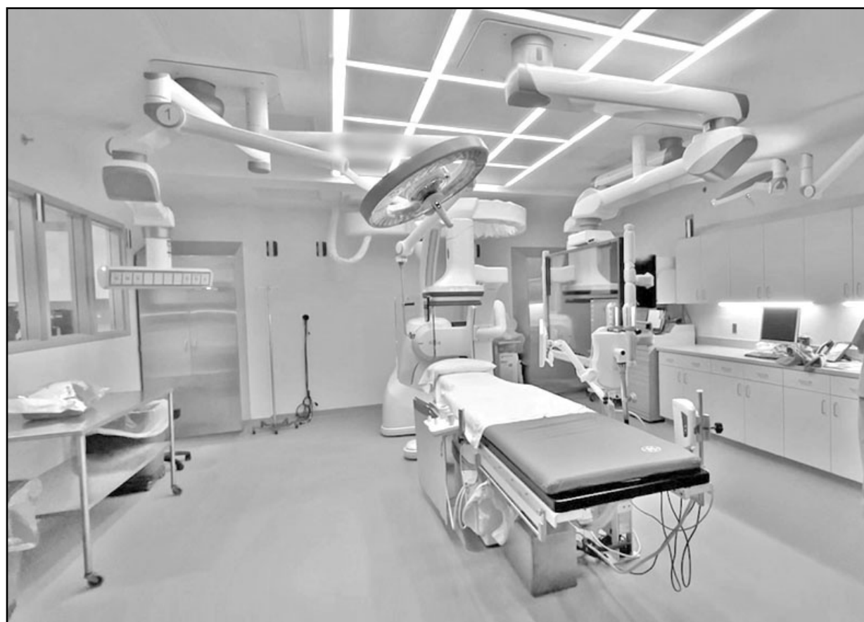
LewisGale Medical Center's state-of-the-art cardiovascular catheterization lab provides advanced treatments that make complex procedures safer and simpler.
