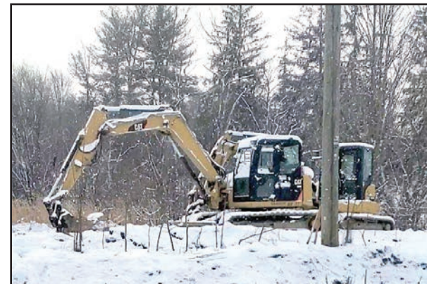
Construction was at a standstill during the Thursday morning snowstorm, but is still expected to be completed within their 120 day estimate.
