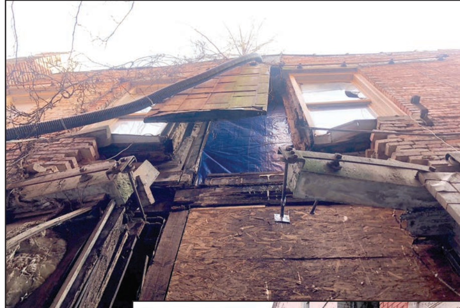
Under the collapsed Rexall wall
