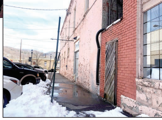
An alternate drainage pipe from the Rexall roof is diverting water outside of the alley to the sidewalk.
