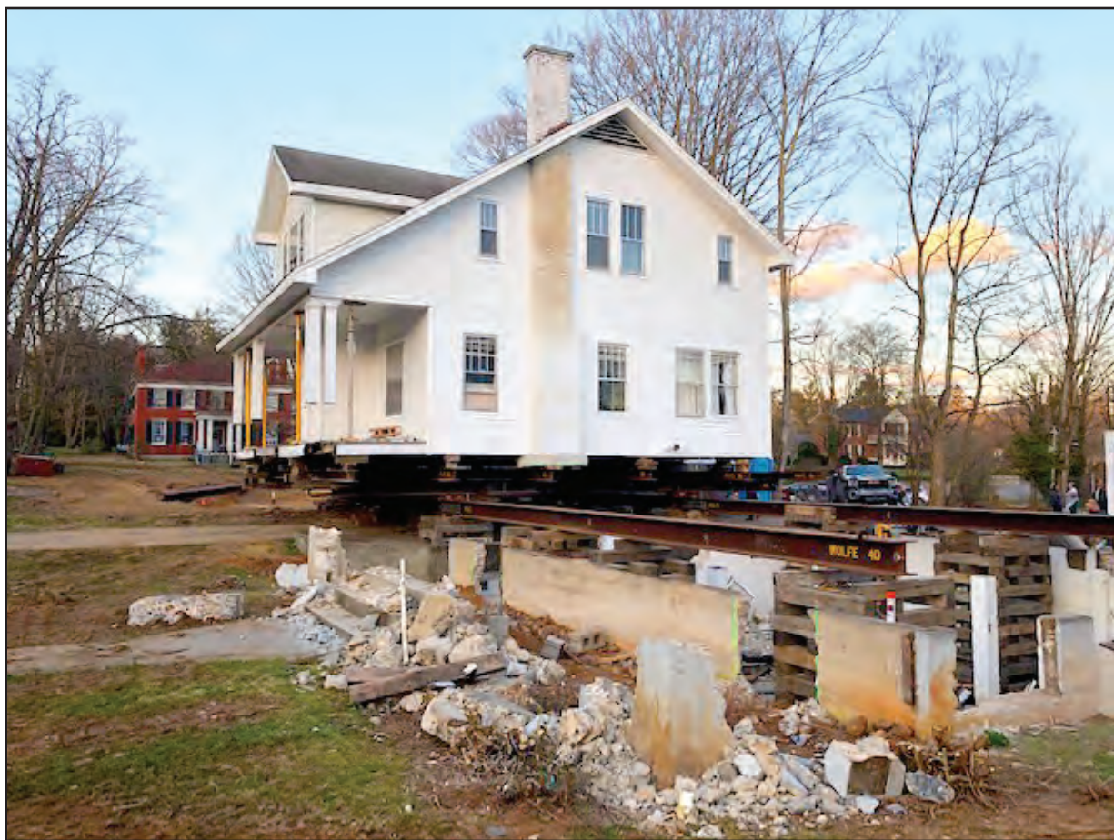
It was a three-day process to gingerly jack up the house and relocate it approximately 100 feet to the left. (Photo by William "Skip" Deegans)
