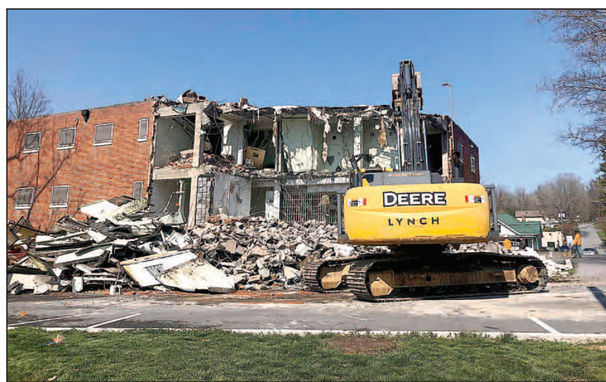
The removal of the old jailhouse will leave only the foundation when all's said and done.
