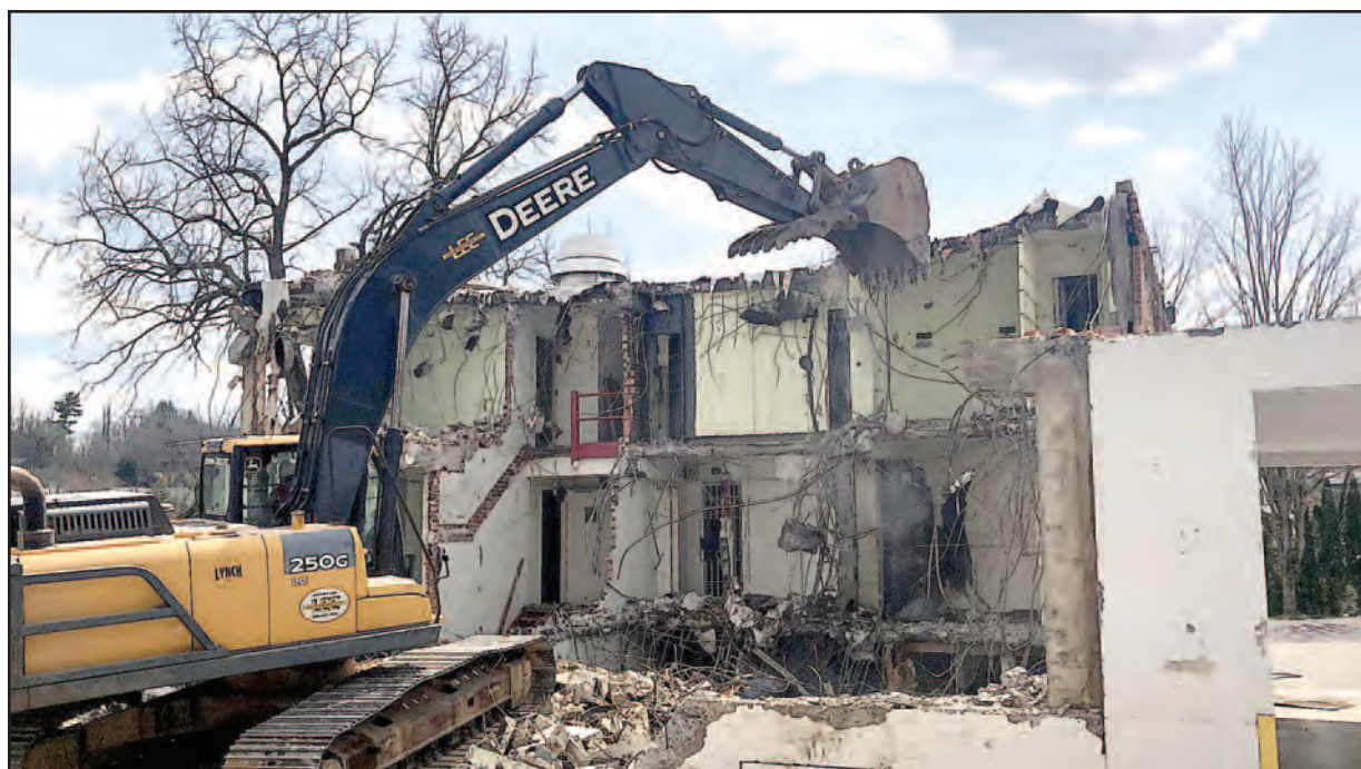
The old structure was not in great condition and needed removed in order to make room for courthouse improvements and expansion.
