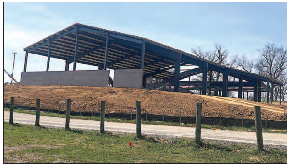
The new roof for the Greenbrier Valley Aquatic Center is the first major physical structure installed for the building.
