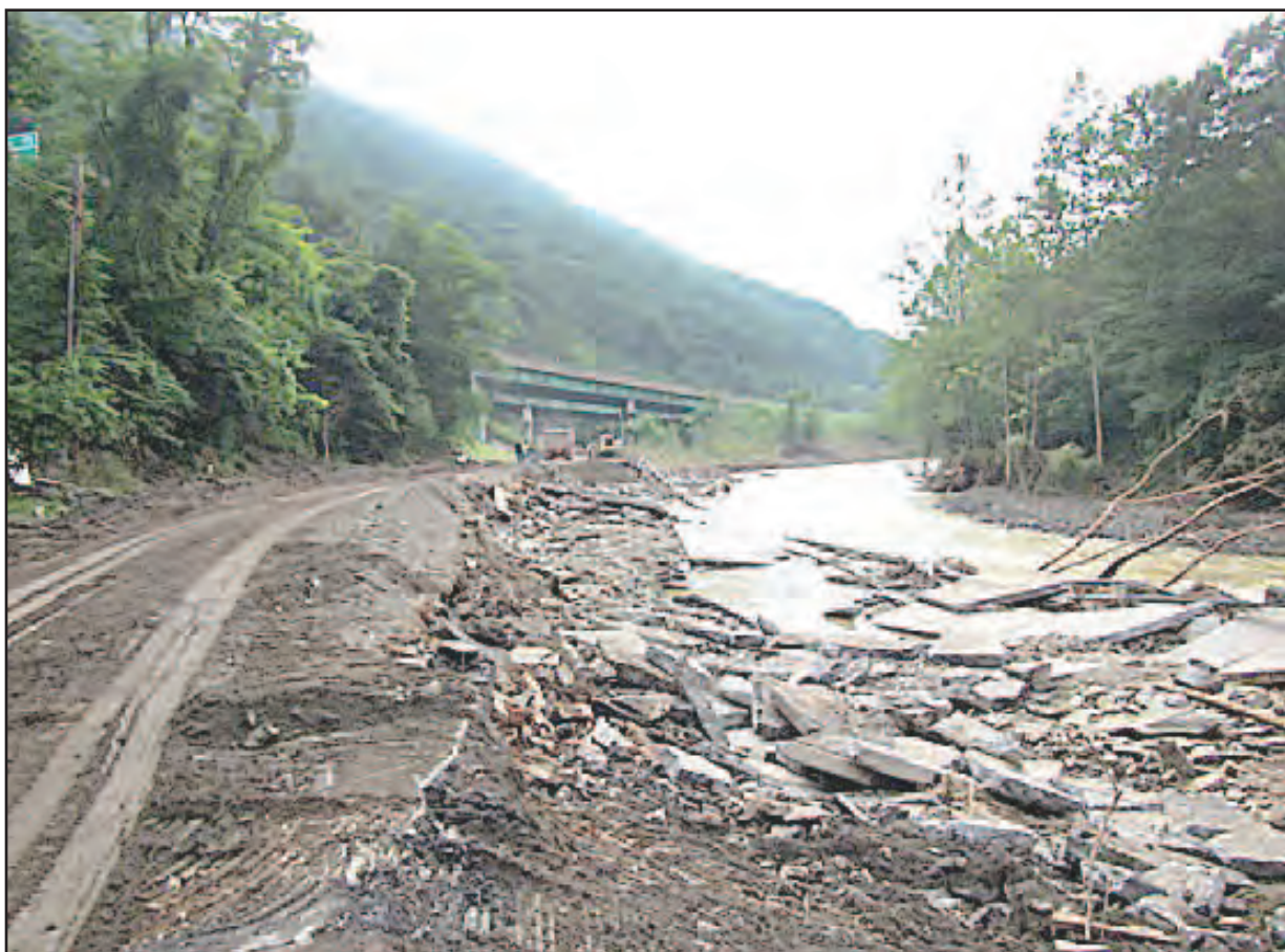
In 2016, Howard's Creek washed out part of Rt. 60 between Caldwell and Harts's Run
