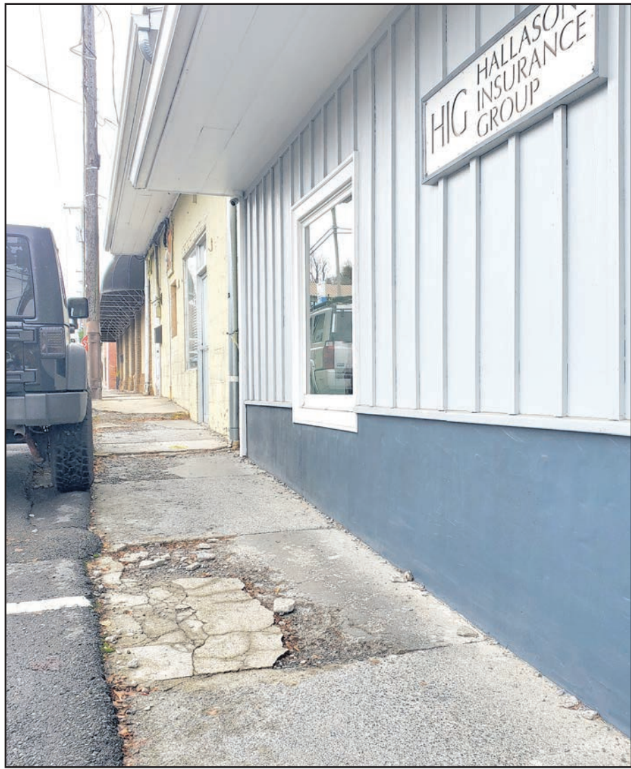
Portion of sidewalk on Lafayette Street in need of repair
